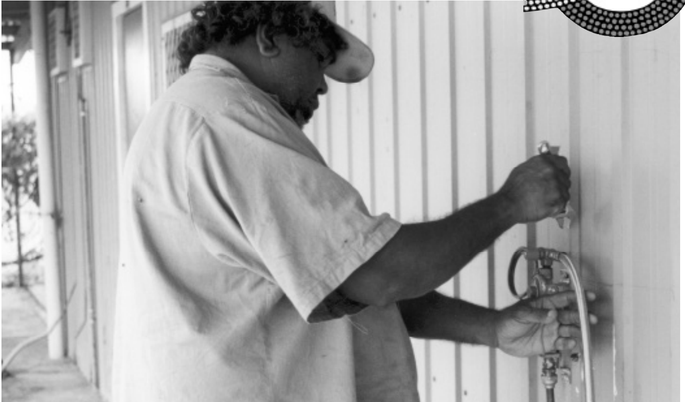
MARK FLY, FIELD OFFICER WITH TJUWANPA RESOURCE AGENCY INSTALLS A FLEXIBLE PIG TAIL FITTING.
