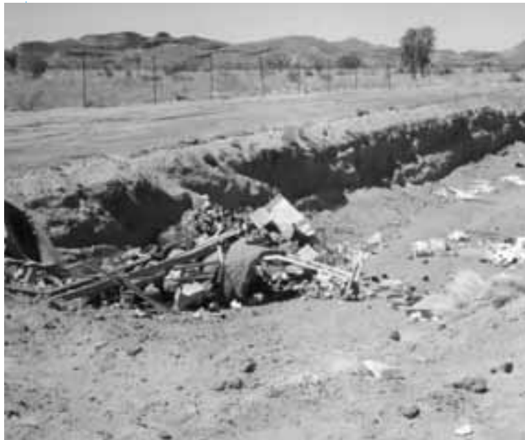
THE TRENCH METHOD OF LANDFILLING REPRESENTS GOOD VALUE FOR MONEY FOR ARID REGIONS. IT IS NOT SUITABLE FOR TROPICAL REGIONS, WHERE WASTE SHOULD BE DEPOSITED IN ABOVE-GROUND CELLS.
